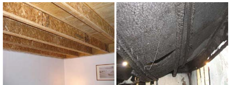
Composite wood joists before (left) and after fire exposure. Photo credit: Tyco Fire Suppression and Building Products
